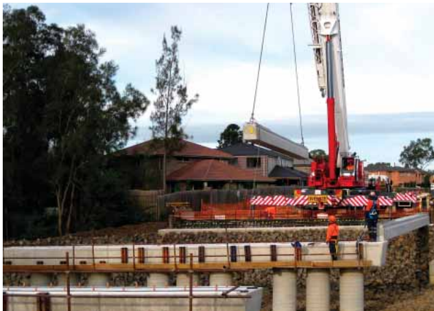
A crane lifts planks into position on Hinchinbrook Bridge, Hoxton Park Road.
