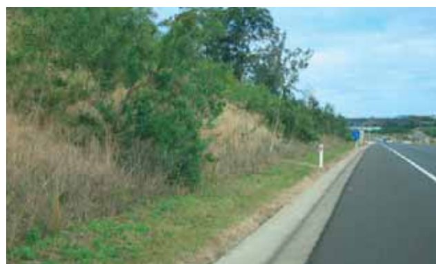
Vegetation growth on the Bonville Bypass, Pacific Highway, in June 2010, just two years after opening.
