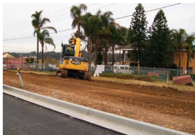
Excavators trim the verges on Camden Valley Way between Bernera Road and Cowpasture Road.
